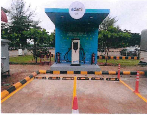
Electric vehicle charging station
